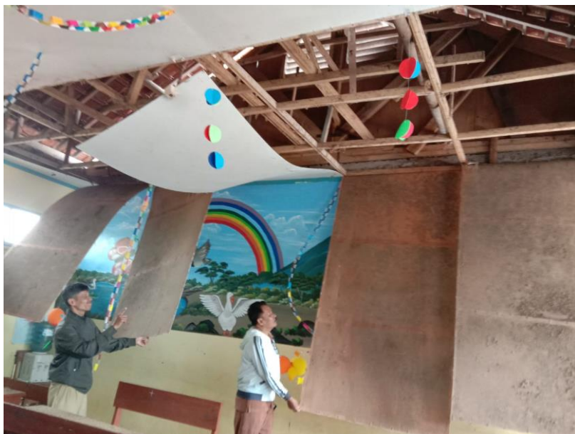
Part of the ceiling came down in the school during the earthquake. Luckily no children were around when it happened
